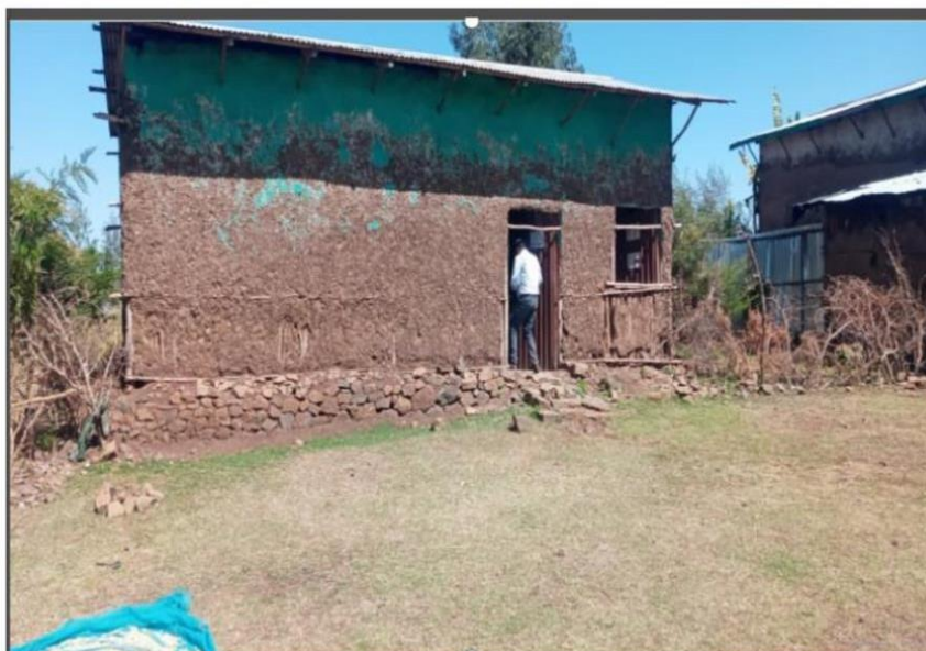
Figure 4: A building that is not satisfactory, at Enemay district
