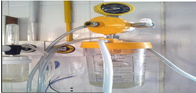
Figure 2: Central suction unit
